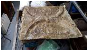
1992.73.1-30 Circa 30 tin ceiling tiles possibly from 1 st Masonic Hall in Quesnel scorching of paint and some rust.
